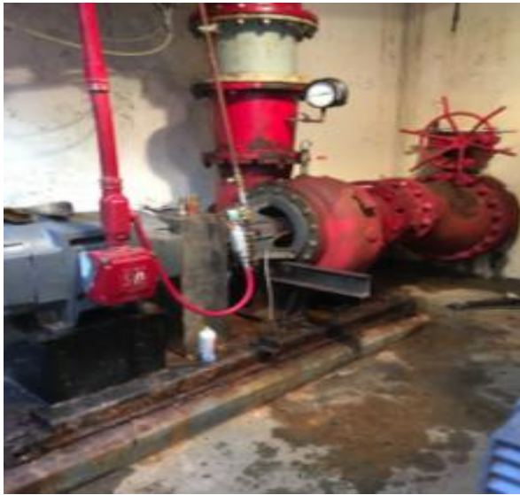
Old Backwash Pump
