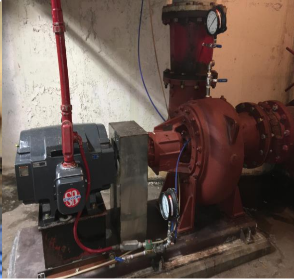
New Backwash Pump
