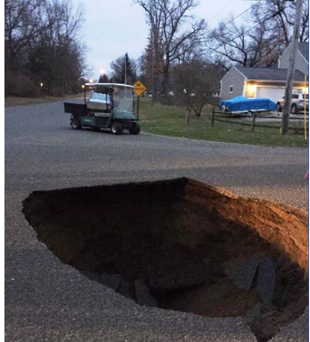
March 27 sewer collapse near Gary Lane and Ann Drive. Emergency repairs such as this can be expensive. Photo from Facebook; photographer unknown.
